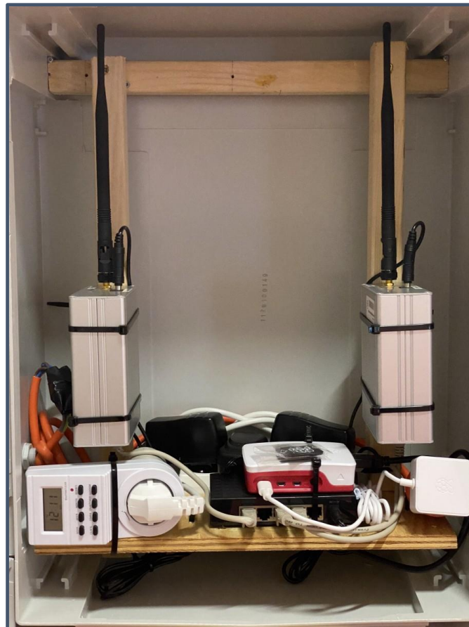
Fig. 1: Components inside the LoRa sniffer box
